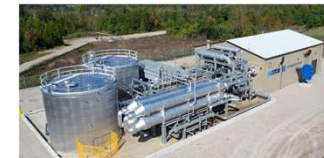
Compressed Air Energy Storage
