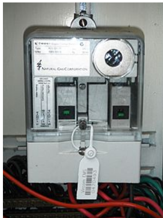
Ripple injection receiver Uses pulses on the lines to control load
