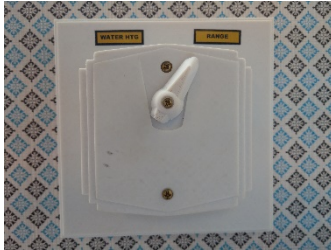
2 position switch Water Heater OR Range
