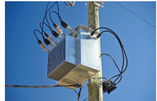
Distribution to low voltage
