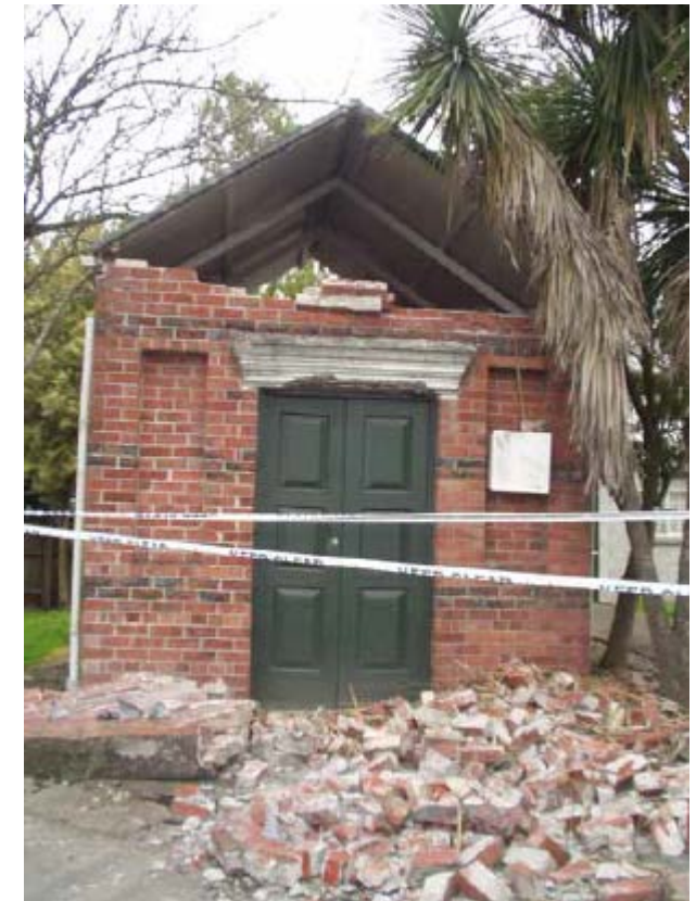
No Seismic Strengthening
