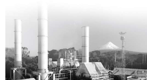
UPDATE Gas Transmission Security and Reliability Update March 2017
