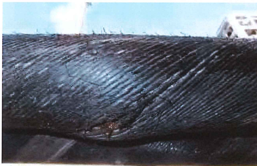
Figure 8. Damaged Basslink cable, 2016. The exact cause of the damage is still being contested as of in February 2017. (Photo provided by Basslink to news media.)
