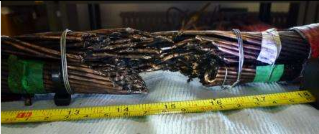
Figure 18 Failed Remuera K 10 joint: arc crater in three conductors after cleaning and re-assembly
