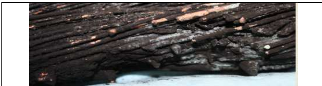
Figure 78 Arc crater: 33 kV XLPE, Carbine Road 2, 2EY, 72.8 m
