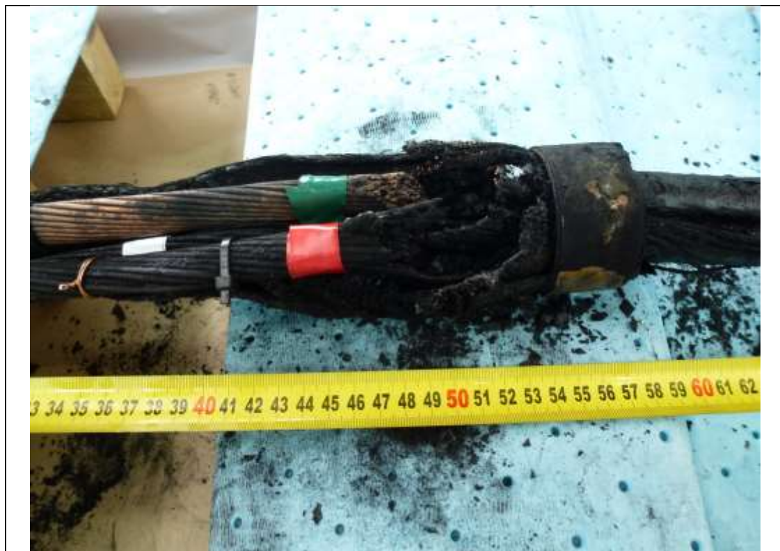
Figure 17 Failed joint: arc crater in the three conductors
