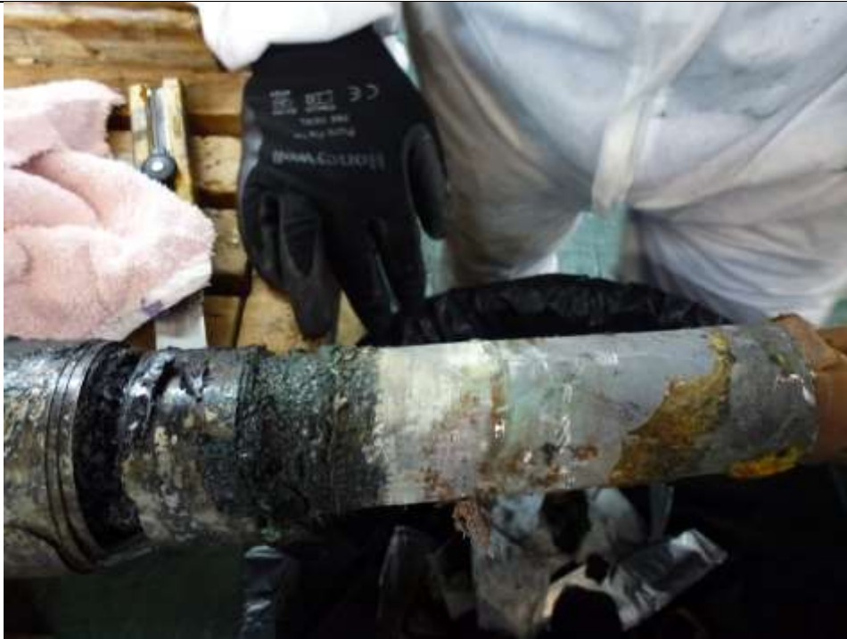
Figure 32 White corrosion products at the current contact with the lead sheath
