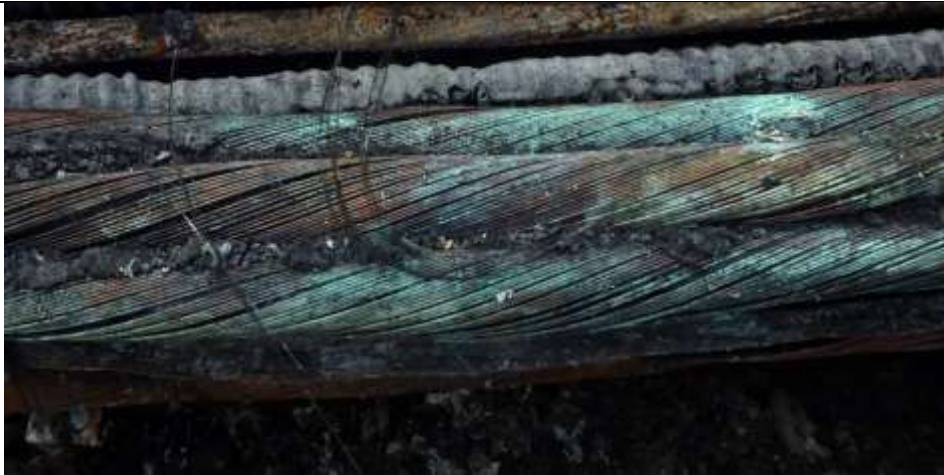
Figure 54 Heat deformed and ruptured OF cable corrugated aluminium sheath
