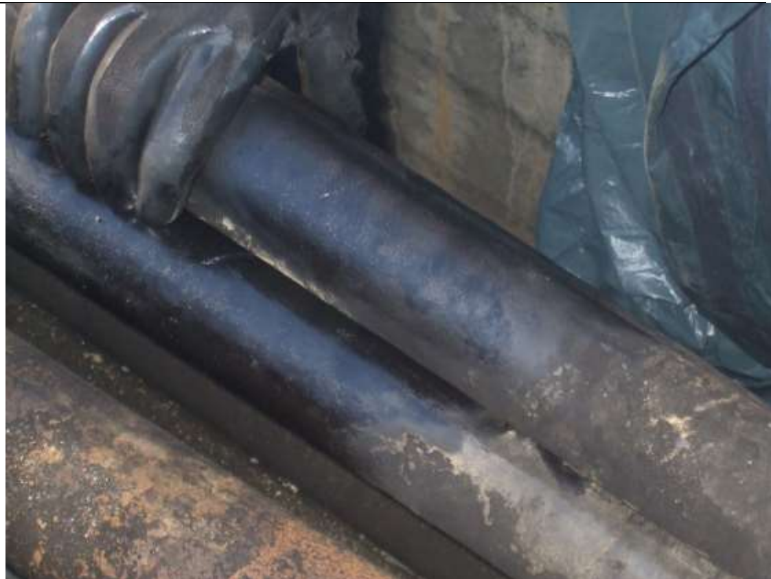
Figure 15 Char of the PE oversheath on Level 1 at 20.3 m
