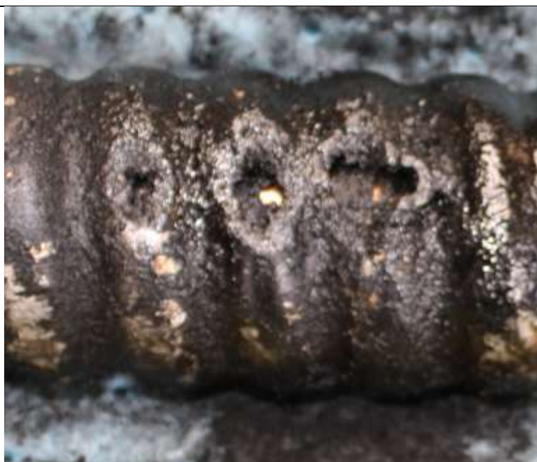
Figure 53 Holes in OF cable aluminium sheath, cable 2D0 at 66-71m
