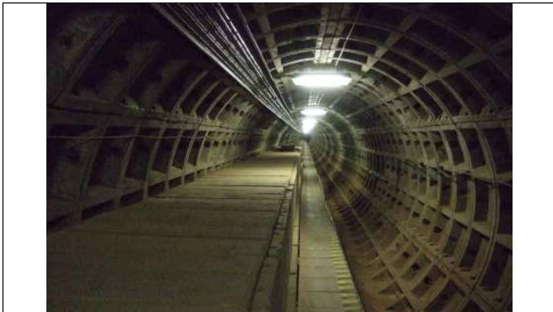
Figure 130 Wimbledon tunnel containing a cable trough
