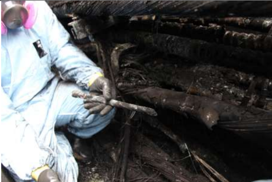
Figure 13 The severed conductor from the Remuera K10 transition joint
