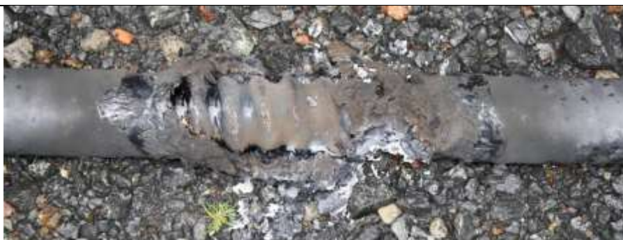
Figure 51 33 kV OF cable: oversheath burnt and aluminium sheath melted
