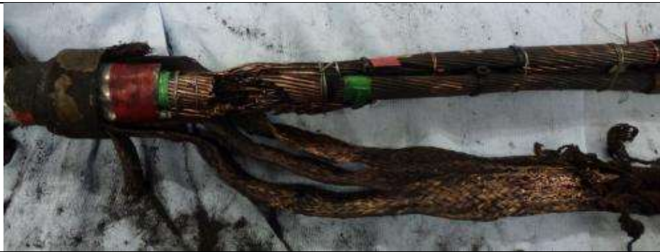
Figure 19 Failed joint: Arc burning to the earth continuity braided conductors
