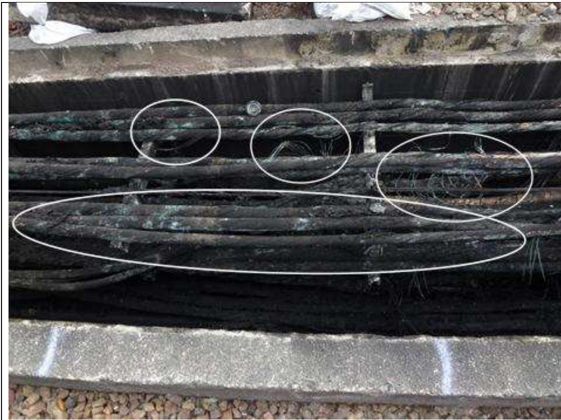
Figure 9 Disturbance indicative of violent electrical activity at 72 m- 74 m
