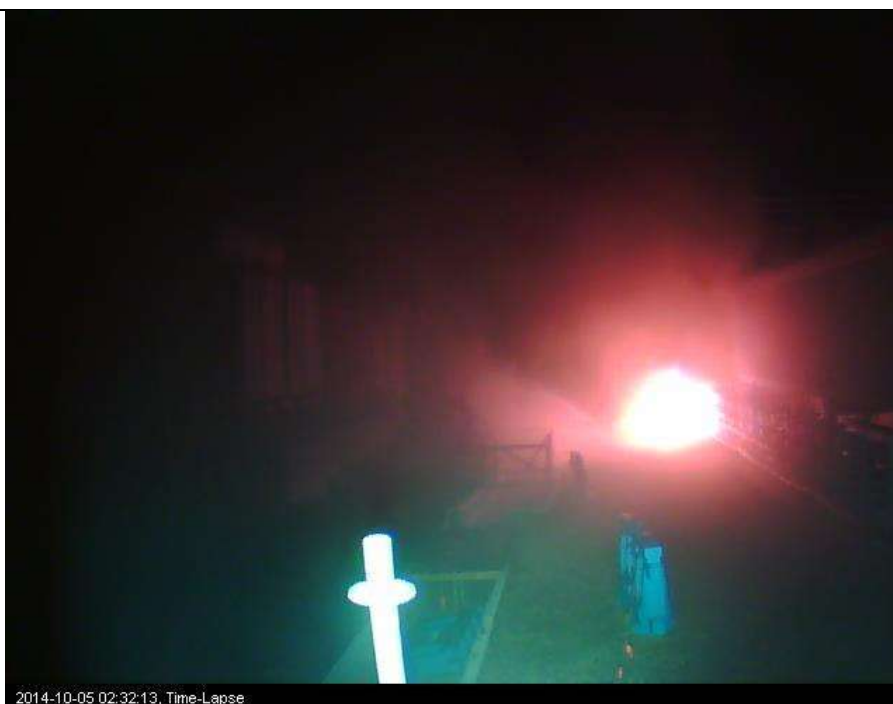
Figure 59 CCTV at 02:32:13, 250.72 m after 1 st fault, 131.4m after 2 nd : Free fire from trench exit close to 33 kV Switchroom corner. Dense smoke
