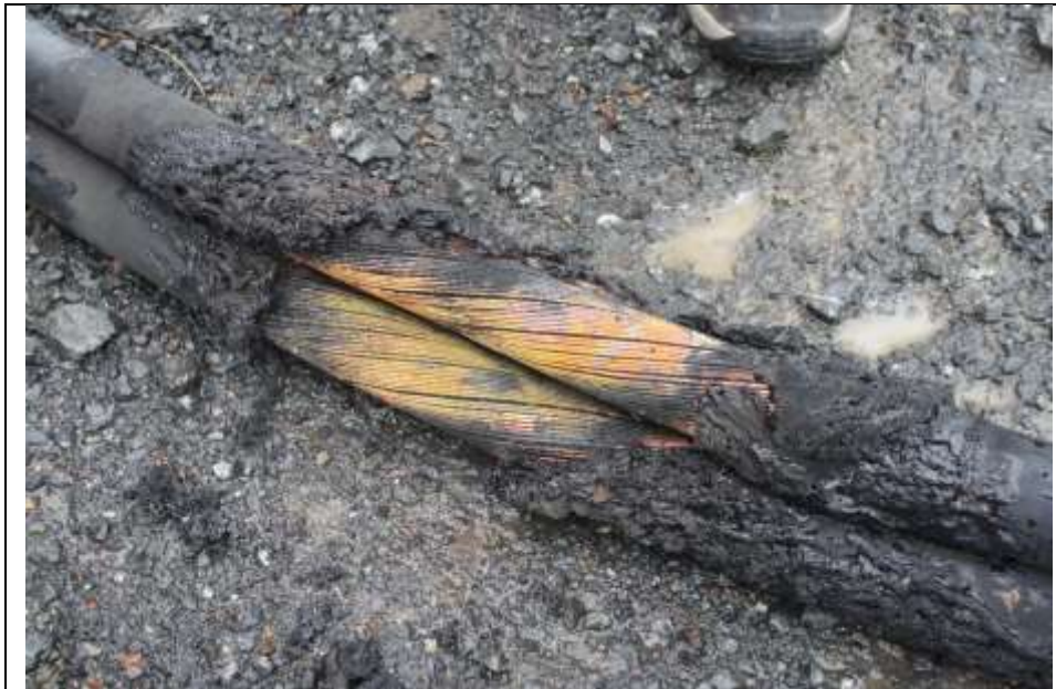
Figure 49 33 kV XLPE trefoil group: oversheath combusted
