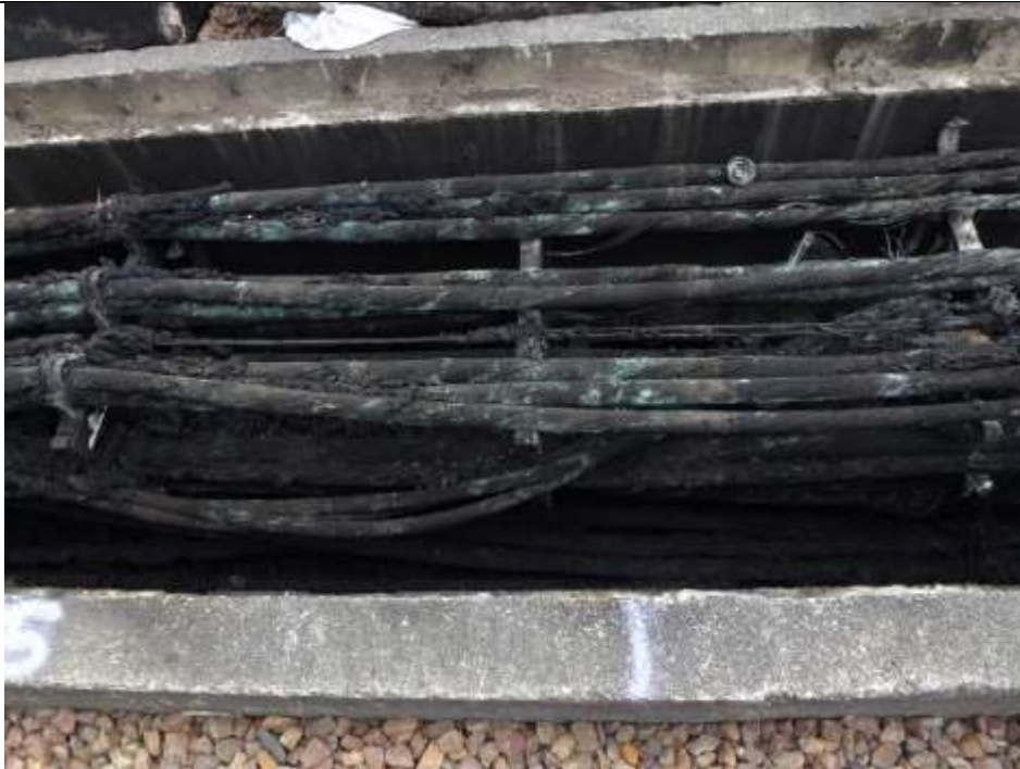
Figure 42 Bow shape in the 11 kV three core XLPE cable between 73 m and 77 m chainage
