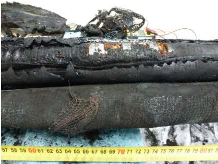
Figure 24 Unfailed joint. Fire damage to the heat-shrink insulation package The outer protective heat shrink sleeve was removed to reveal the internal joint components, Figure 25.
