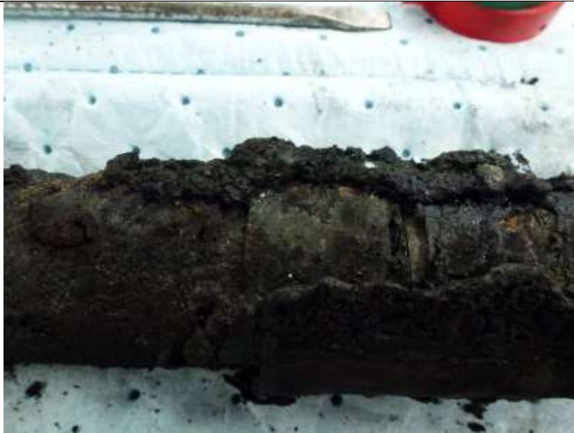
Figure 23 Unfailed joint. The steel roll springs could be seen on the PILC side The fire has also burnt along the central heat shrink packages to varying degrees to reveal part of the bimetallic connectors, Figure 24.
