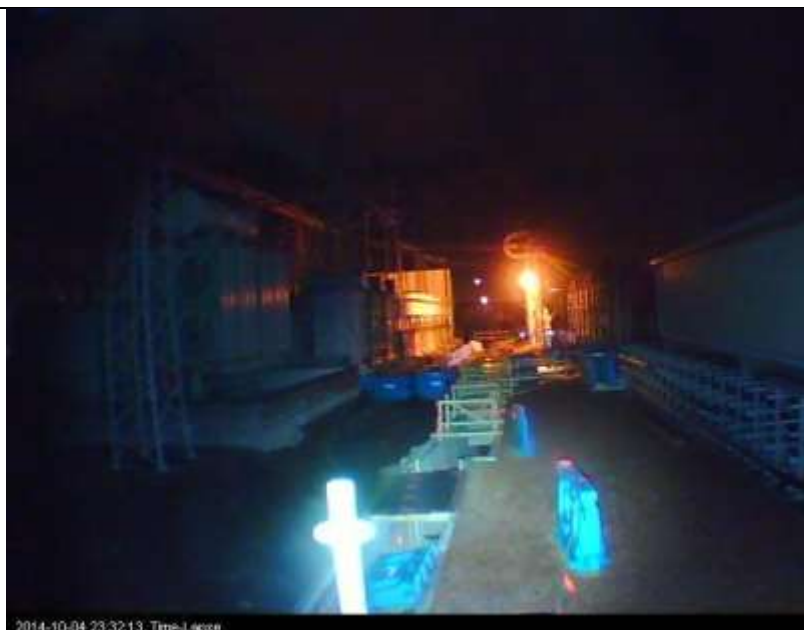
Figure 56 CCTV at 00:32:13, 70.72 m after 1 st fault: view of T11 and T10 become obscured. Reflection on T10 obscured view of reflection obscured dull reflection off T11
