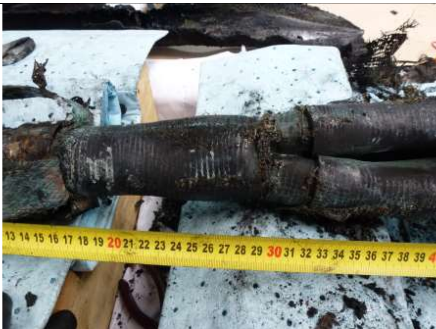
Figure 26 Unfailed joint. The heat shrink 'break-out' covering the PILC crutch
