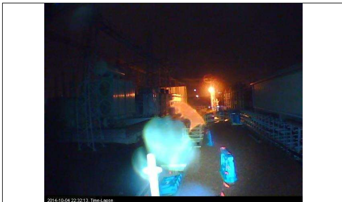
Figure 55 CCTV at 23:32:13, 10.72 m after 1 st fault: sharp reflections off T11 side and expansion tank and off side of T10
