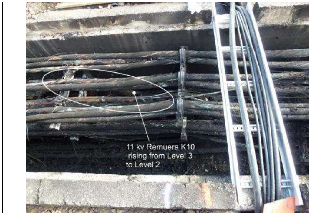
Figure 11 11 kV Remuera K10 cable rising from Level 3 to Level 2
