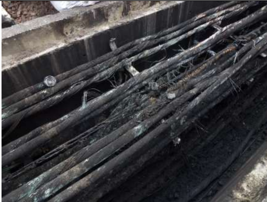
Figure 8 Photograph of cable trench at 73 m taken after the fire in October 2014
