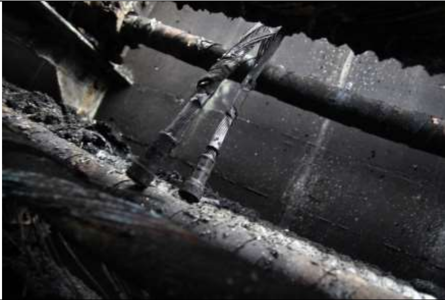
Figure 12 Two parted conductors hanging from the failed transition joint
