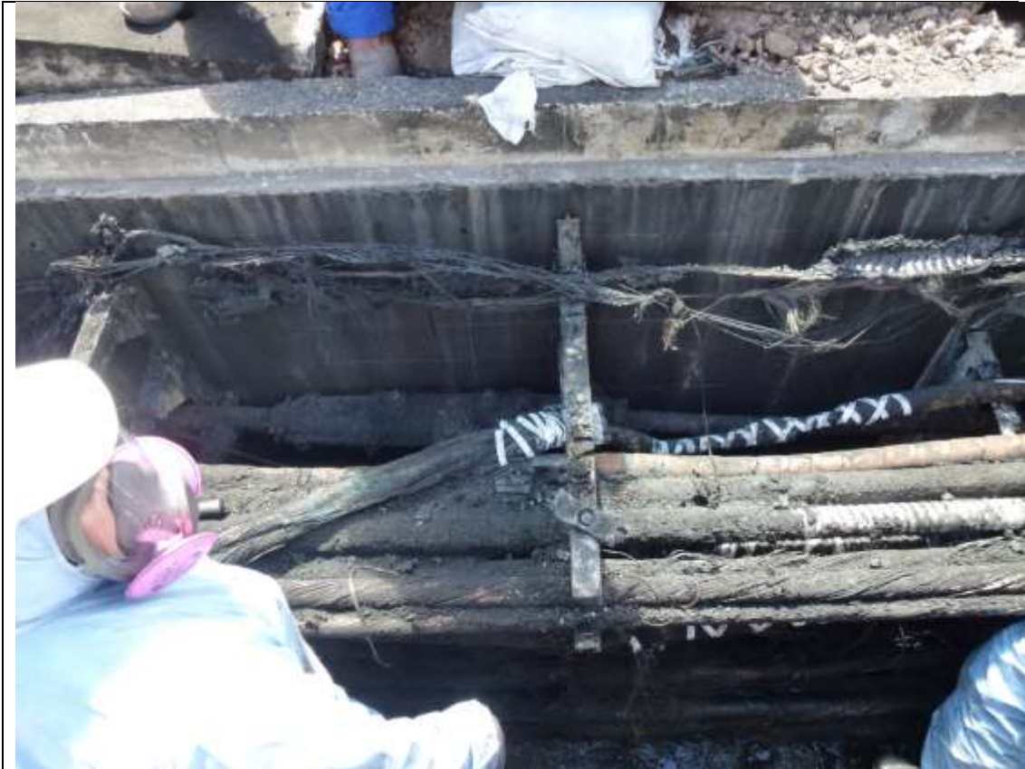
Figure 14 Level 1 cables removed to reveal the failed transition joint on Level 2 and a conventional cast-iron joint below it on Level 3
