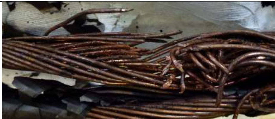
Figure 92 Arc crater: 11 kV PILC, Mt Wellington K05, 4D0
