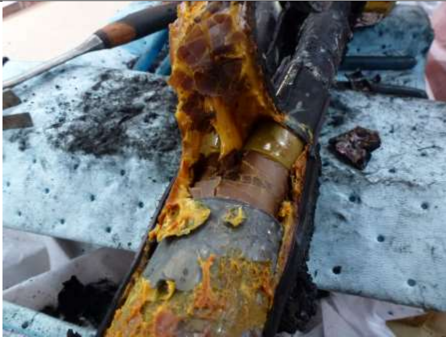
Figure 29 The mastic had not uniformly adhered to the lead sheath
