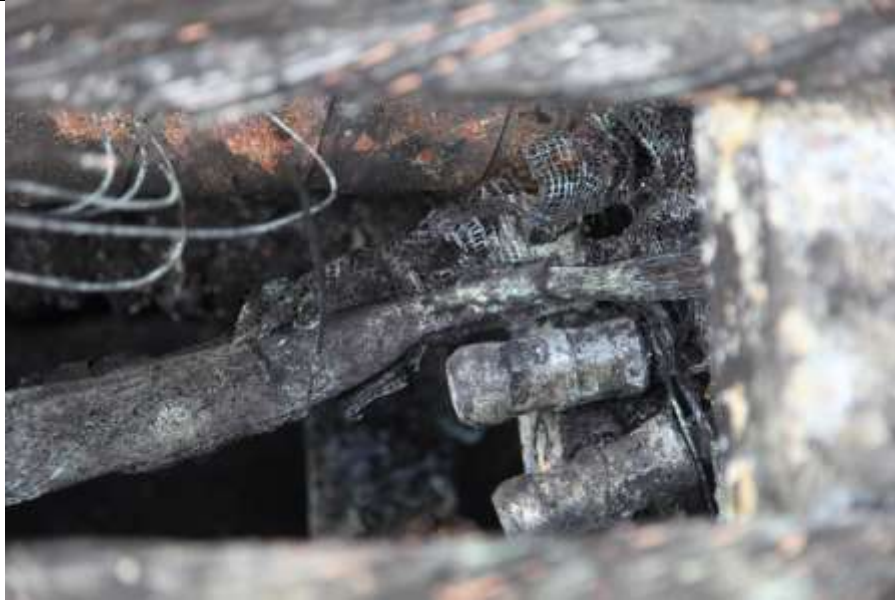
Figure 10. Close view of failed transition joint between cable Layers 1 and 2
