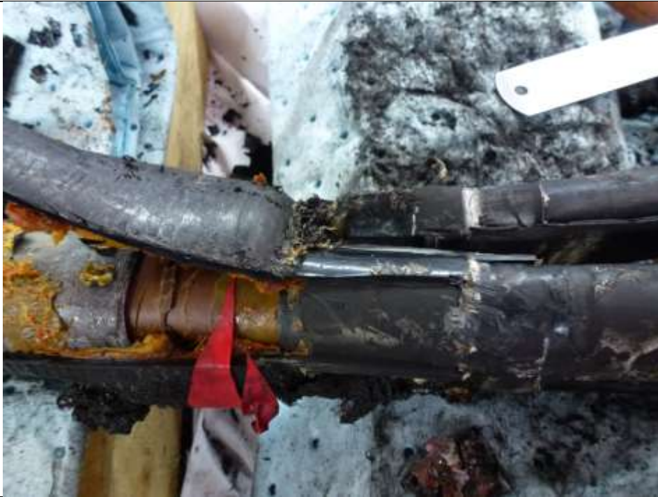
Figure 28 Unfailed joint. Arc centre is in PILC crutch close to oil barrier sleeve
