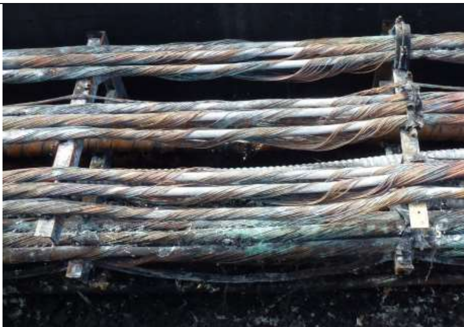
Figure 52 High fire intensity at 37 m (33 kV XLPE cables on top Level)
