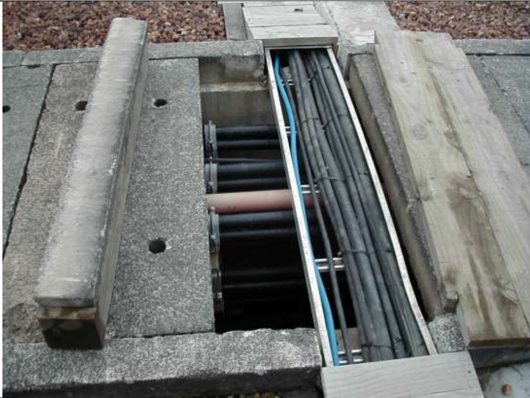
Figure 44 Control cable bridge at 70.5 m (photo taken in 2001)
