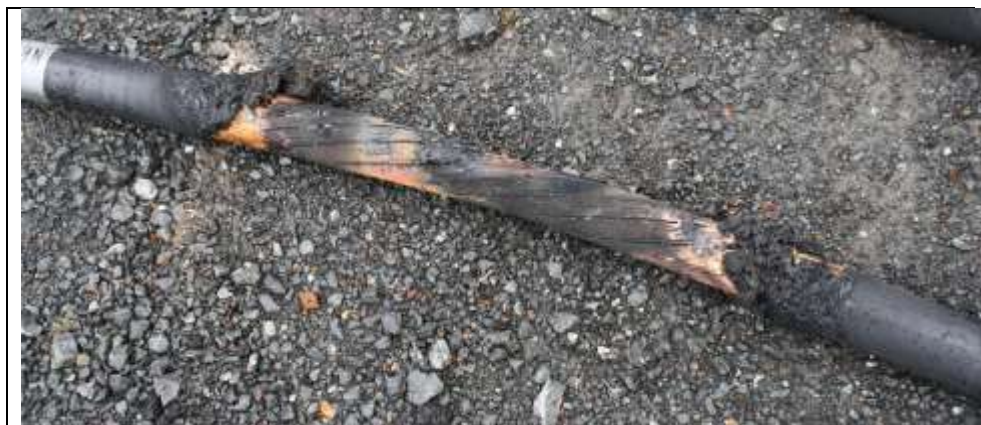
Figure 47 33 kV XLPE cable: oversheath combusted
