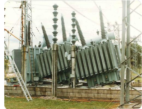
Transformer damage Edgecumbe 1987
