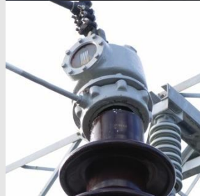
Failure of two HV bushings on T2 (66kV/11kV)
