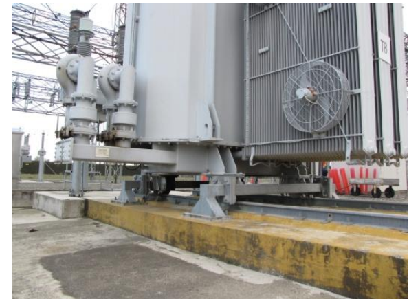
Transformer seismic restraints Hororata
