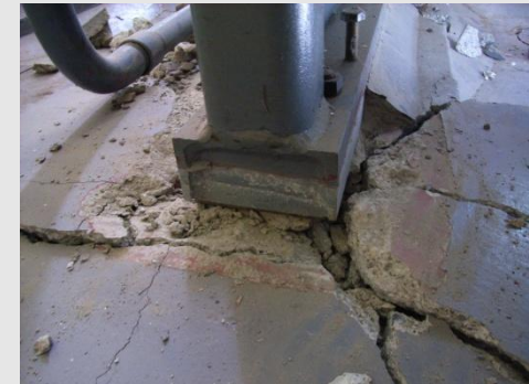
Damage to 11 kV switchboard; remained operational during the event – is being replaced
