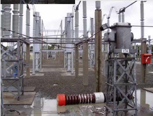
Failure of one 220 kV CVT BRY-ISL1 RFS
