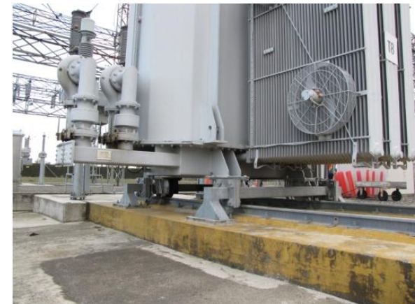
Transformer seismic restraints Hororata
