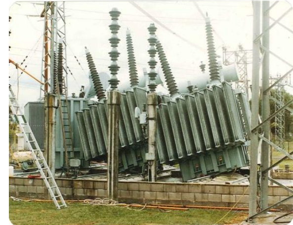
Transformer damage Edgecumbe 1987
